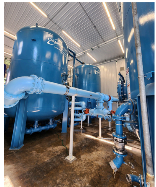
Shown here are the Waterloo Water Treatment Plant's Calgon Carbon filters that take out contaminants from Seneca Lake water
