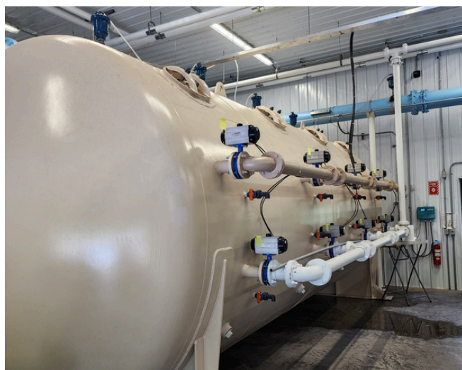
The Waterloo Water Treatment Plant's tan tanks are Horizontal Pressure Filters (HPFs) that filter out dirt and algae from Seneca Lake water for municipal use.
